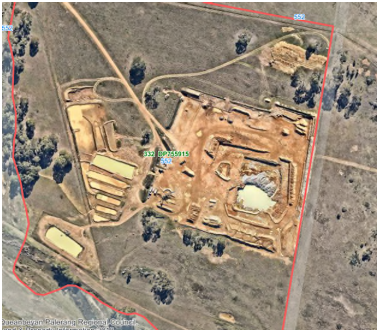
Figure 4 – Current operations showing unauthorised work outside the approved extraction area – Nearmap July 2026
