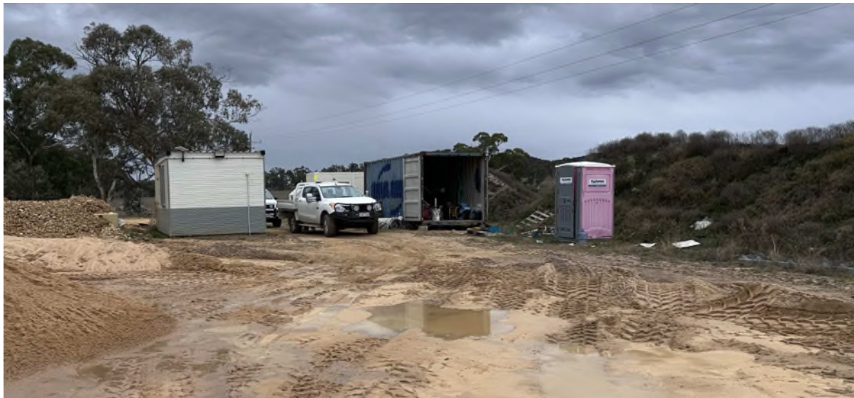
Figure 15: Site shed, storage container located outside the existing approved area. Clearing of topsoil and overburden storage.
